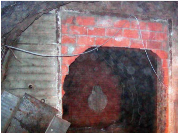
Fig. 13 Masonry wall after explosion [2]
